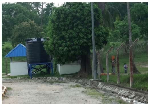
Figure 2: Sample water tank installed to boost local water supply
